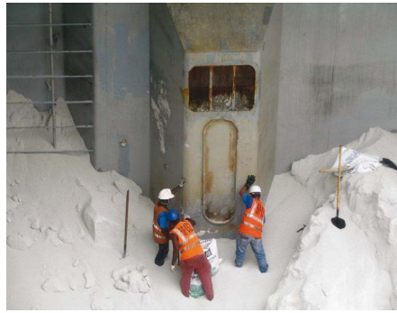
Removing damaged product from cargo hold
